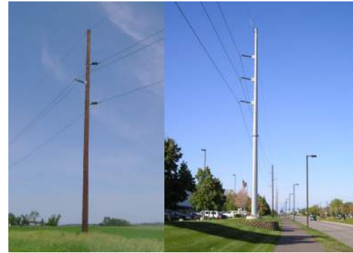
Typical 69-kV single wood structure and steel structure.
