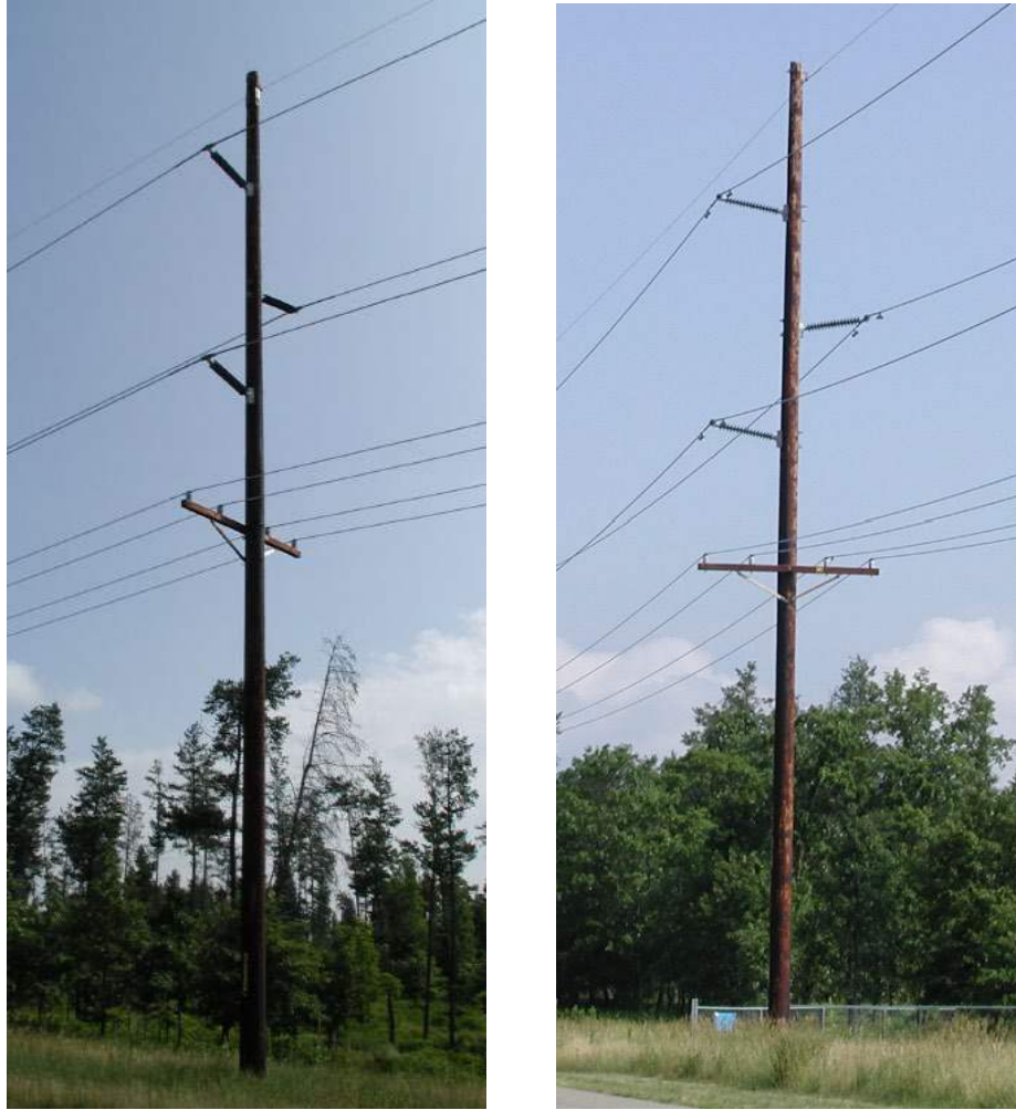
Figure 6 Photos of 115-kV Structures with 3-Phase Distribution Underbuild
