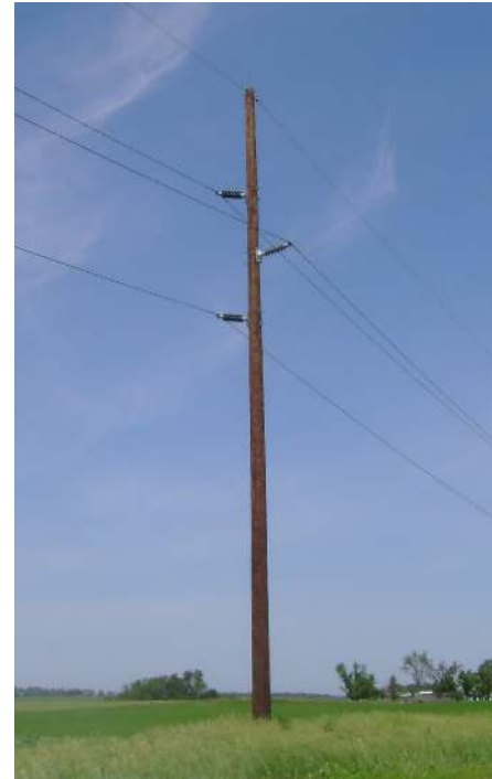
Typical 69-kV single circuit structure
