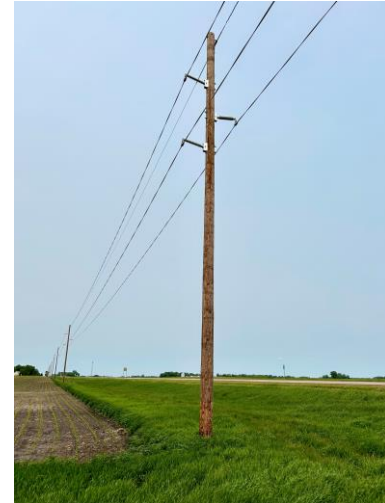
Typical 69-kV single circuit structure
