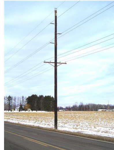
Typical 69-kV wood single circuit structure with distribution underbuild.
