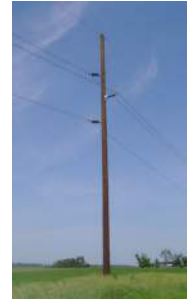
Typical 69-kV wood structure.
