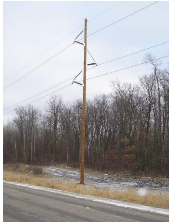
Typical 115-kV single circuit structure
