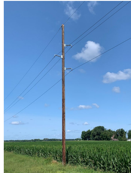
Typical 69-kV wood single circuit structure without distribution underbuild
