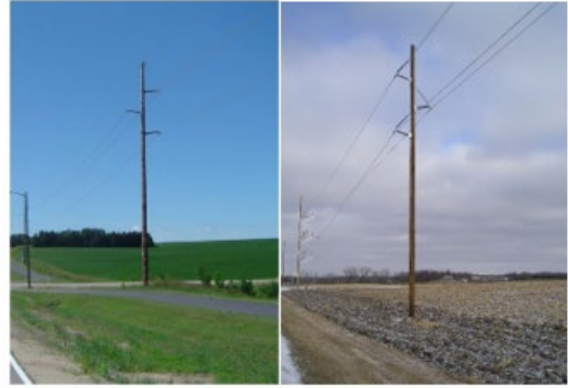
Typical 115-kV single circuit structure and 115-kV with braced posts.
