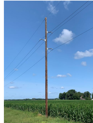
Typical 69-kV wood structure
