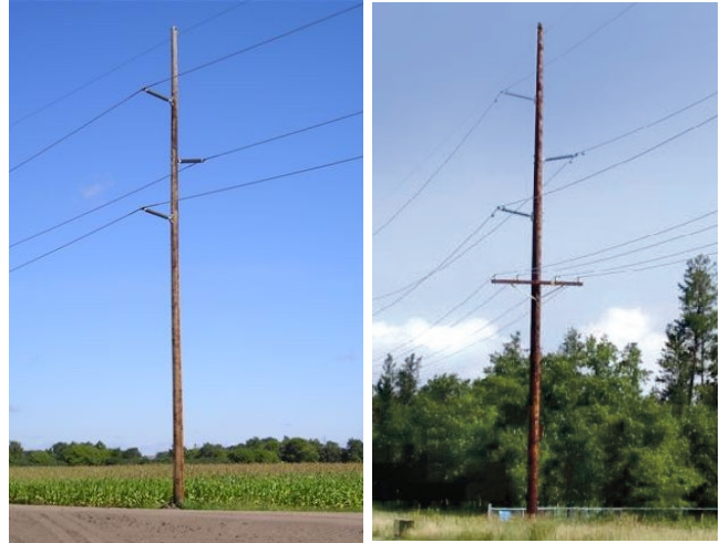
Typical 115-kV single circuit structure with and without distribution under build.
