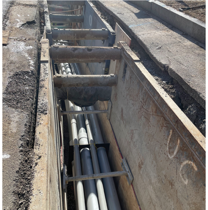
Burying high voltage transmission lines is extremely disruptive to property. An open trench is required throughout the construction process.
