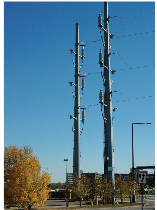
Riser structures are required in some areas when burying transmission lines underground.
