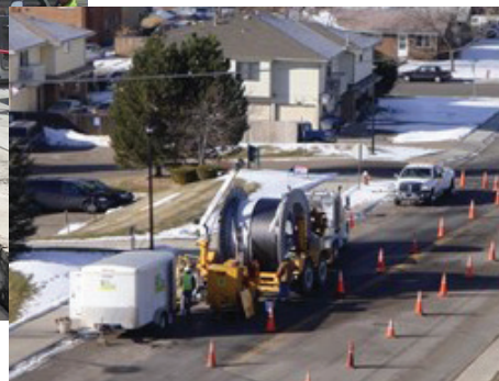
FAR LEFT: A large amount of space is required throughout the construction process while burying transmission lines underground. LEFT: A large section of roadway is blocked off while cables are installed. In urban areas, underdeveloped rights-of-way may require extensive grading to support the construction activities and equipment.
