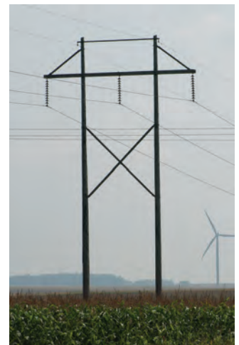
230-kV/345-kV H-frame transmission structure
