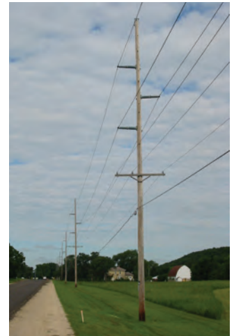
69-kV/115-kV transmission structure with distribution underbuild
