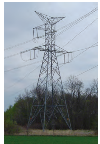
230-kV/345-kV lattice transmission structure
