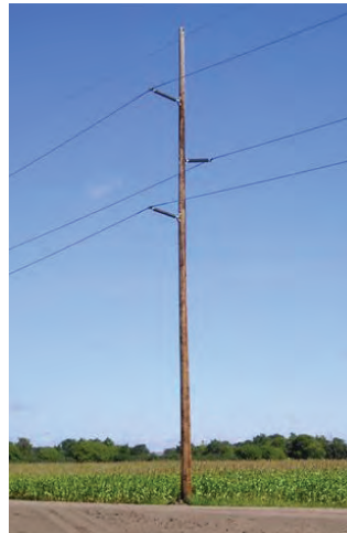
69-kV/115-kV transmission structure
