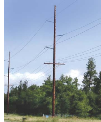
Typical 115 kV wood single circuit structure with distribution underbuild
