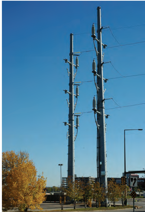
Riser structures are required in some areas when burying transmission lines underground.
