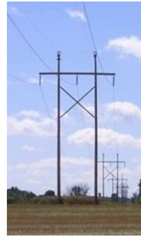
Typical 115-kV H-frame
