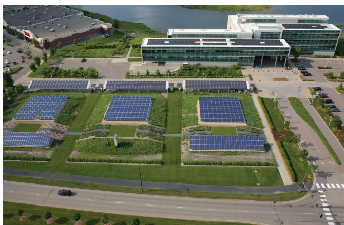
A variety of solar technologies and configurations are being tested at Great River Energy's headquarters site. The 250-kW installation includes panels made by Sharp (two rows pictured at bottom), tenKsolar (three square-shaped clusters) and Suniva (three rows closest to the building).
