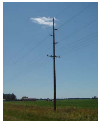
Typical 41.6 kV single-pole wood structure with distribution underbuild
