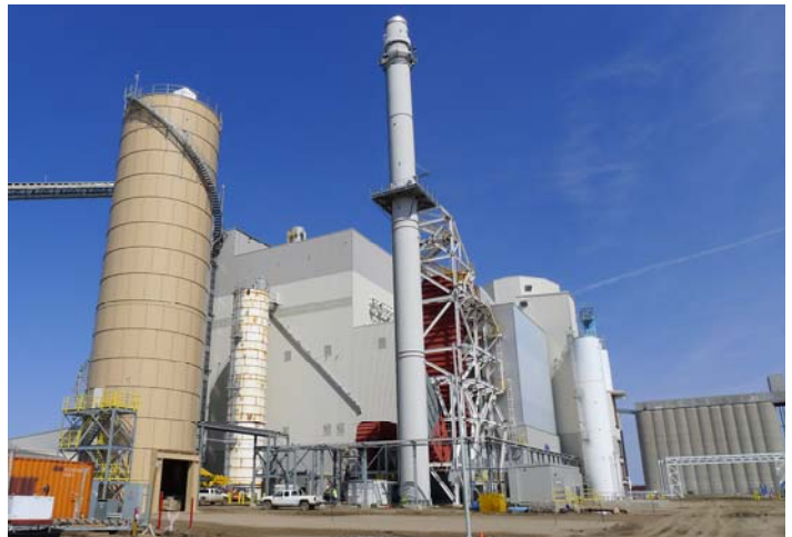
As a combined heat and power plant, Spiritwood Station generates steam and electricity.
